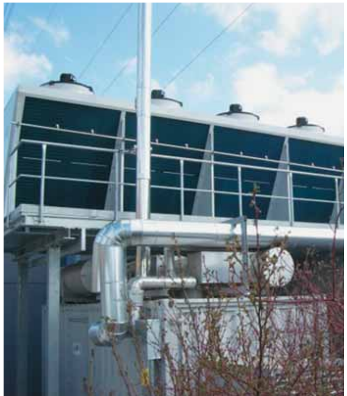
340 kW CHP unit in a container with 220 kW absorption cooler, 50 m 3 vegetable oil tank und two 60 m 3 buffer tanks for heat and cooling energy
