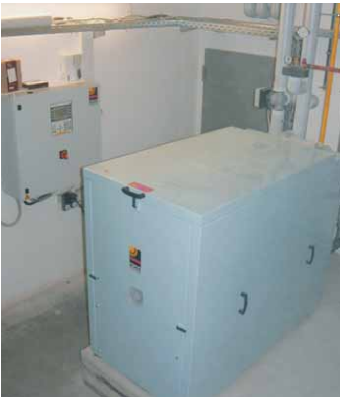
30 kW natural gas powered CHP unit with sound-insulating hood and 2 m 3 buffer tank
