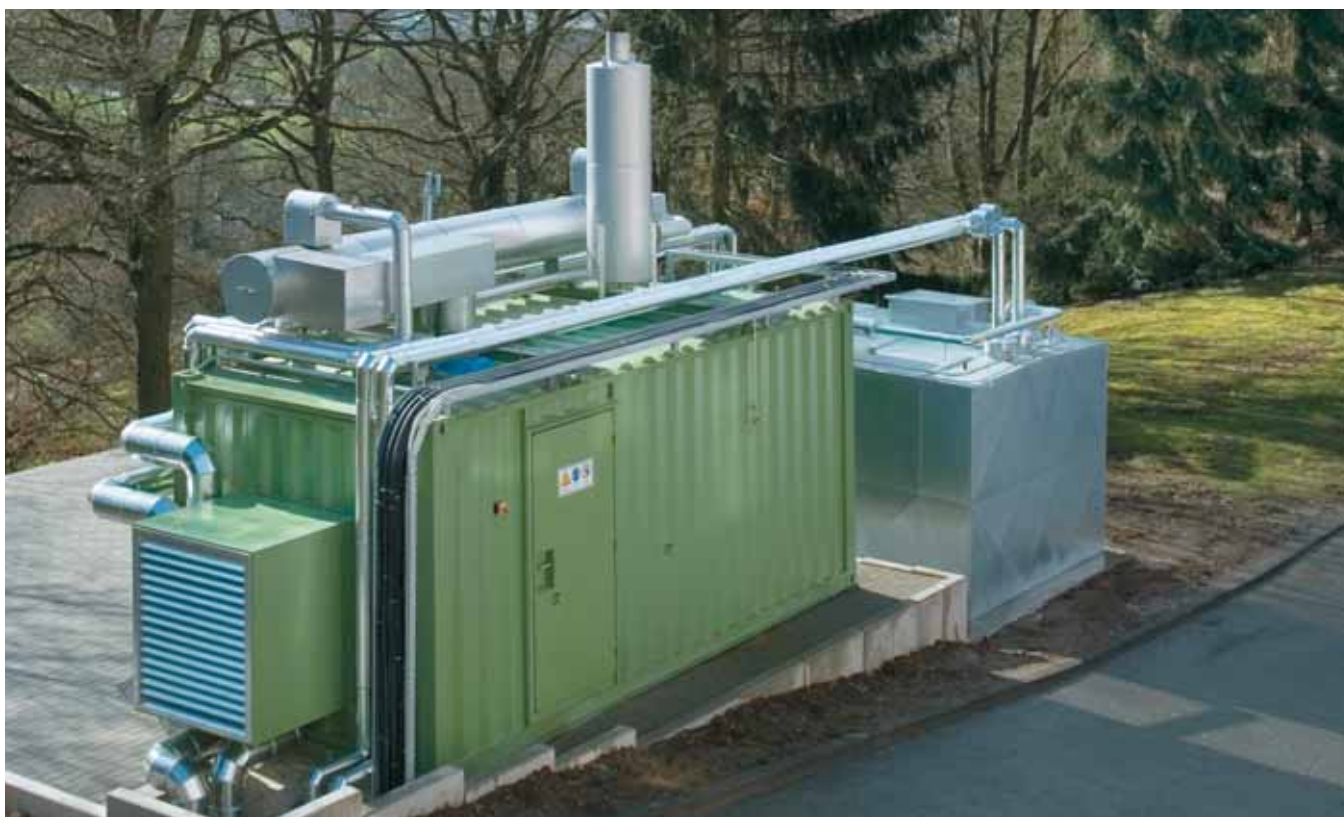
Rittal in Herborn, Germany: 340 KW vegetable oil CHP unit with a Würz 36 m 3 fuel tank.
