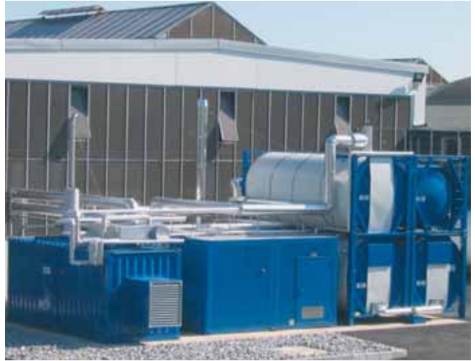
120 kW vegetable oil powered CHP unit in a container with 2 x 24 m 3 vegetable oil tank, heating oil tank with 24 m 3 main tank and 24 m 3 buffer tank
